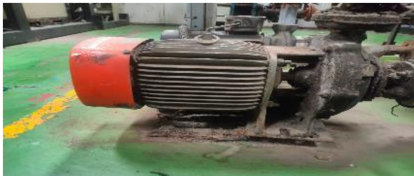
Before- KDI-1000 type, 10 HP two IE1 class induction motors are working for Chiller process water circulation.
