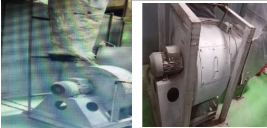
Before- Traditional blower with induction motor was installed in Hard coat -AHU
